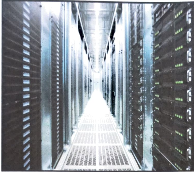
Fig 3.10 Cooling of large data servers
