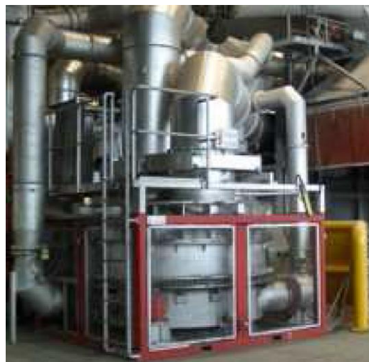
Fig 3.6 Rotary Regenerator on a Melting Furnace
